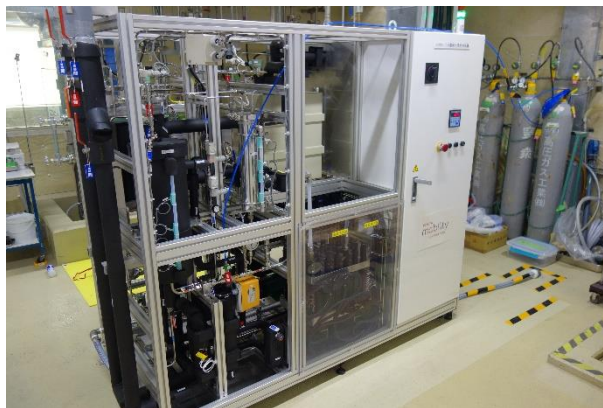
Water electrolysis hydrogen generator
